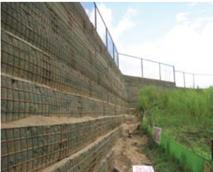
To reach the entire wall with minimal shadowing, crews sprayed from the top down and from the bottom up.
